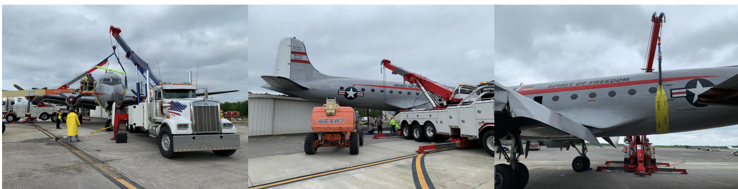
THE REMOVAL OF THE C-54 FROM OFF OF THE HANGAR WAS EXPERTLY PERFORMED BY JASON PENCE AND HIS CREW.
